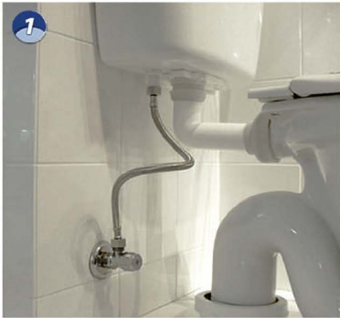
1 Most toilets have a flex pipe.
