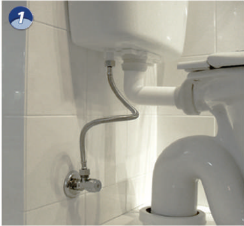
1 Most toilets have a flex pipe.
